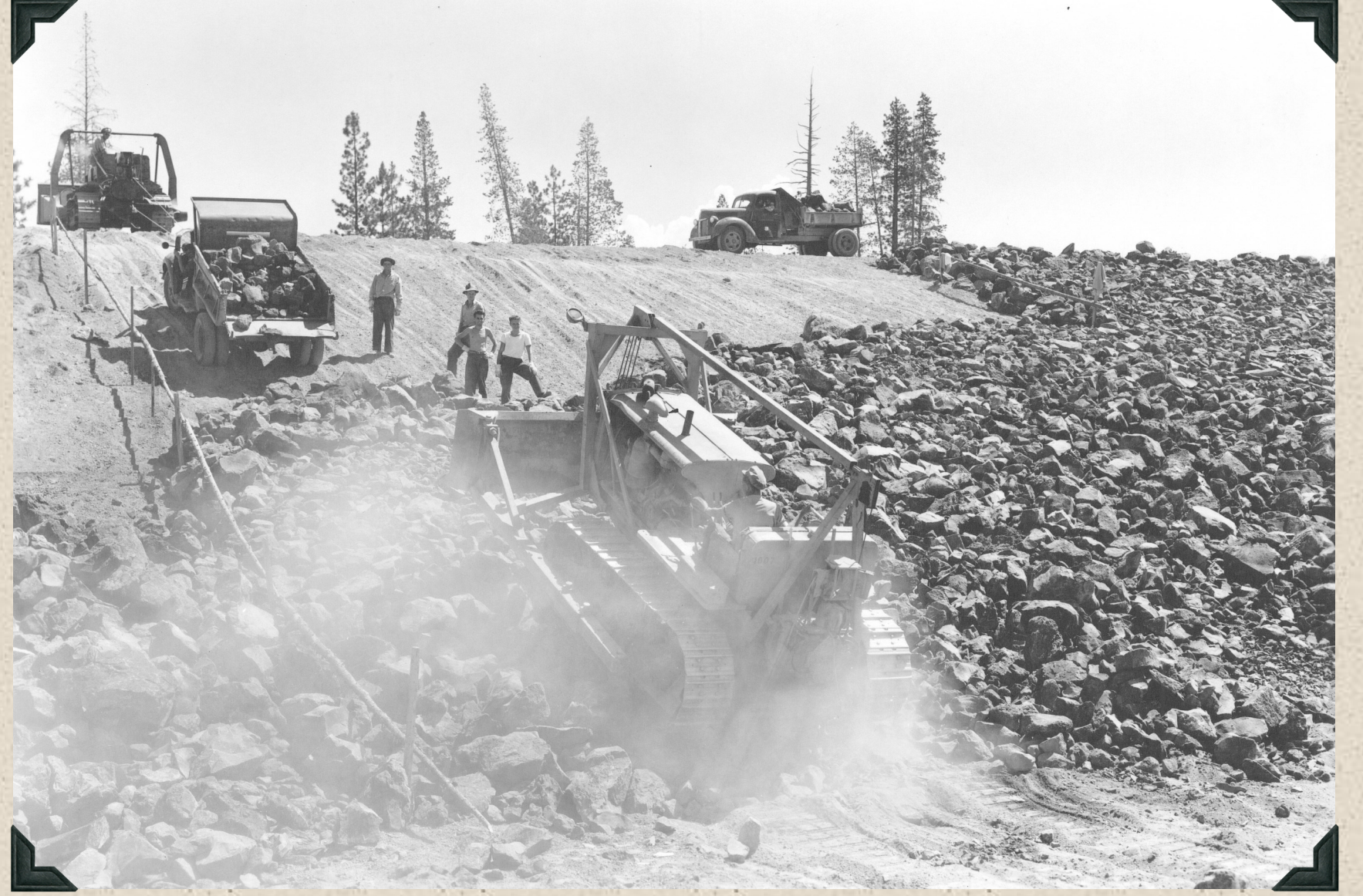
1944 - Wickiup Dam. Civilian Public Service (CPS) assignees placing riprap on upstream face. Dozer shaping toe of riprap.
