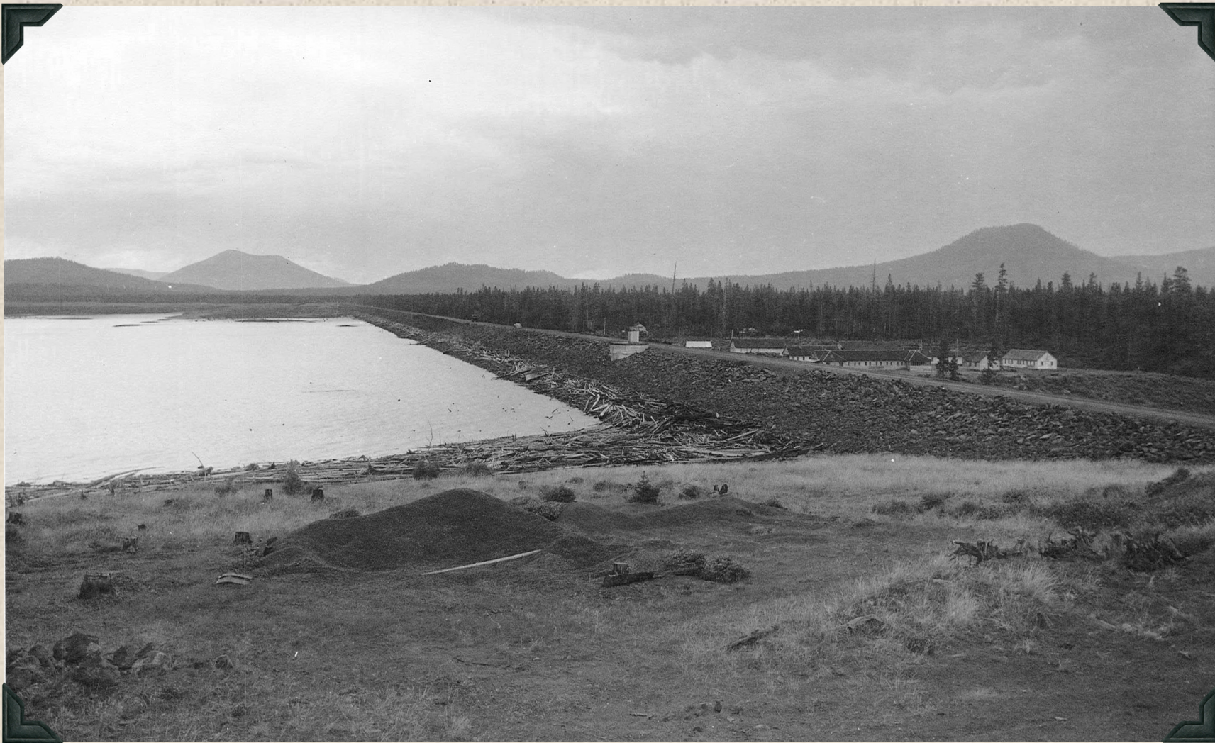
1948 - Wickiup Dam from right bank of reservoir. Dam in process of completion by Adler Construction Co.
