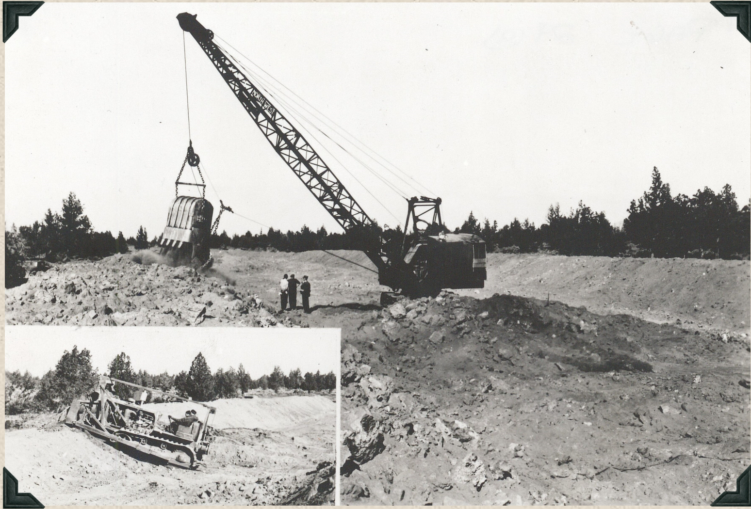
1939 - Dragline excavating of main canal and placing embankment. Inset: Civilian Conservation Corps (CCC) enrollees bulldozer on canal construction.
