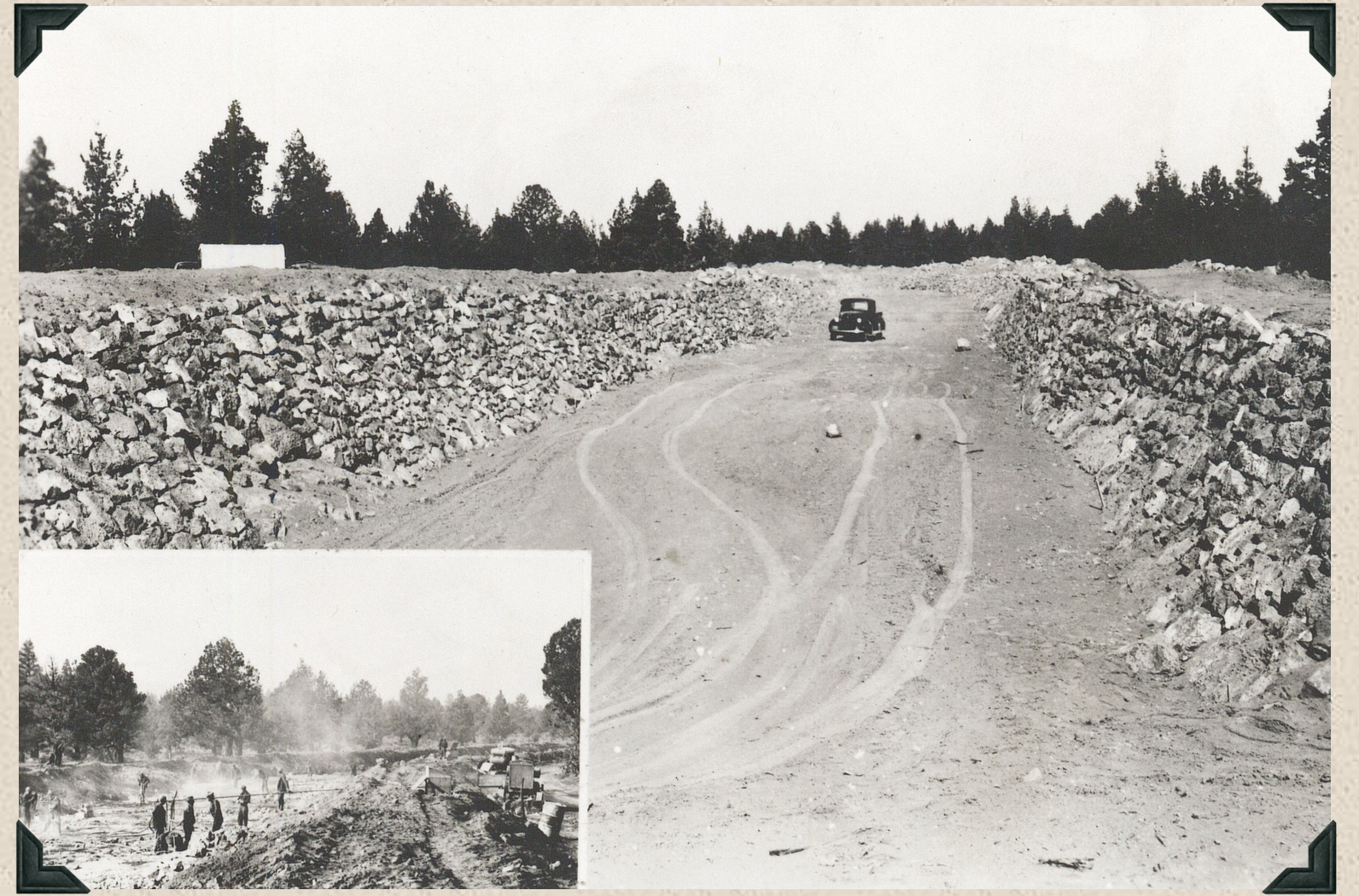
1939 - Completed section of main canal. Inset: Civilian Conservation Corps (CCC) enrollees drilling rock on canal.
