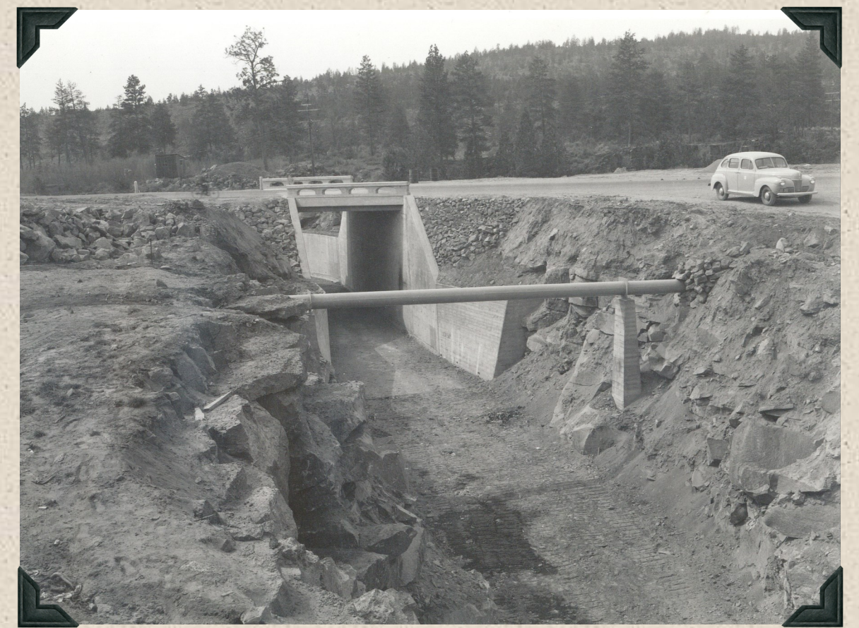
1942 - North Unit Main Canal. Looking upstream from right canal bank. State highway bridge and insulated city water main.
