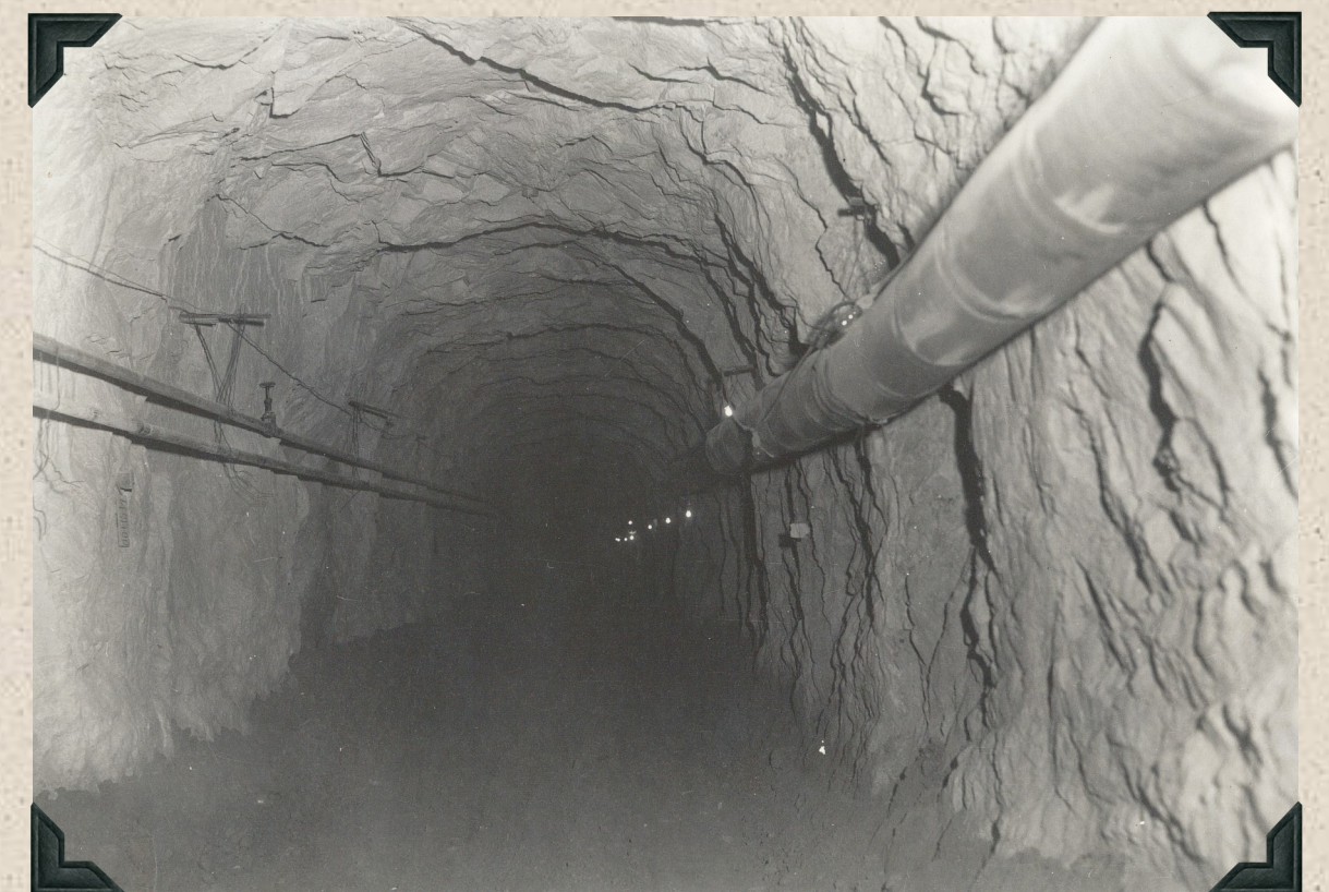
1944 - North Unit Main Canal. View in middle of Tunnel No. 1 showing typical rock formation.
