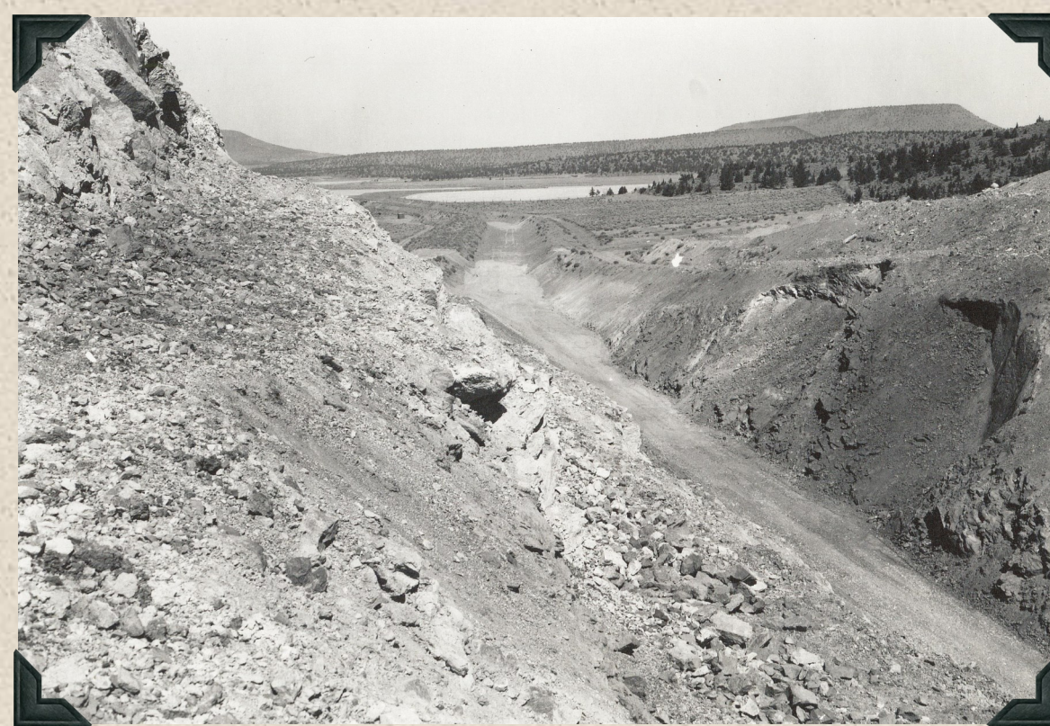
1945 - North Unit Main Canal. View of north end of "Big Cut", looking downstream. (E. B. Bishop, Contractor)
