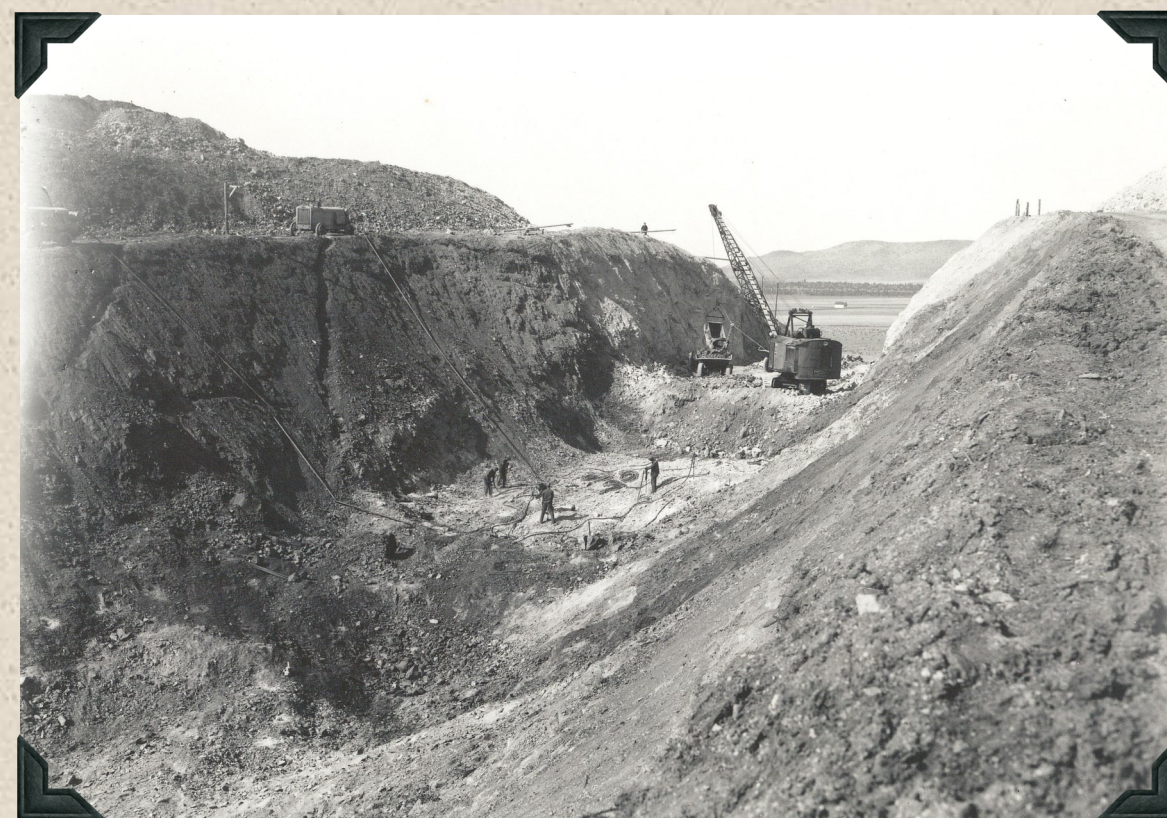
1942 - North Unit Main Canal. Looking downstream from right bank. The "Big Cut", former location of Tunnel No. 3.
