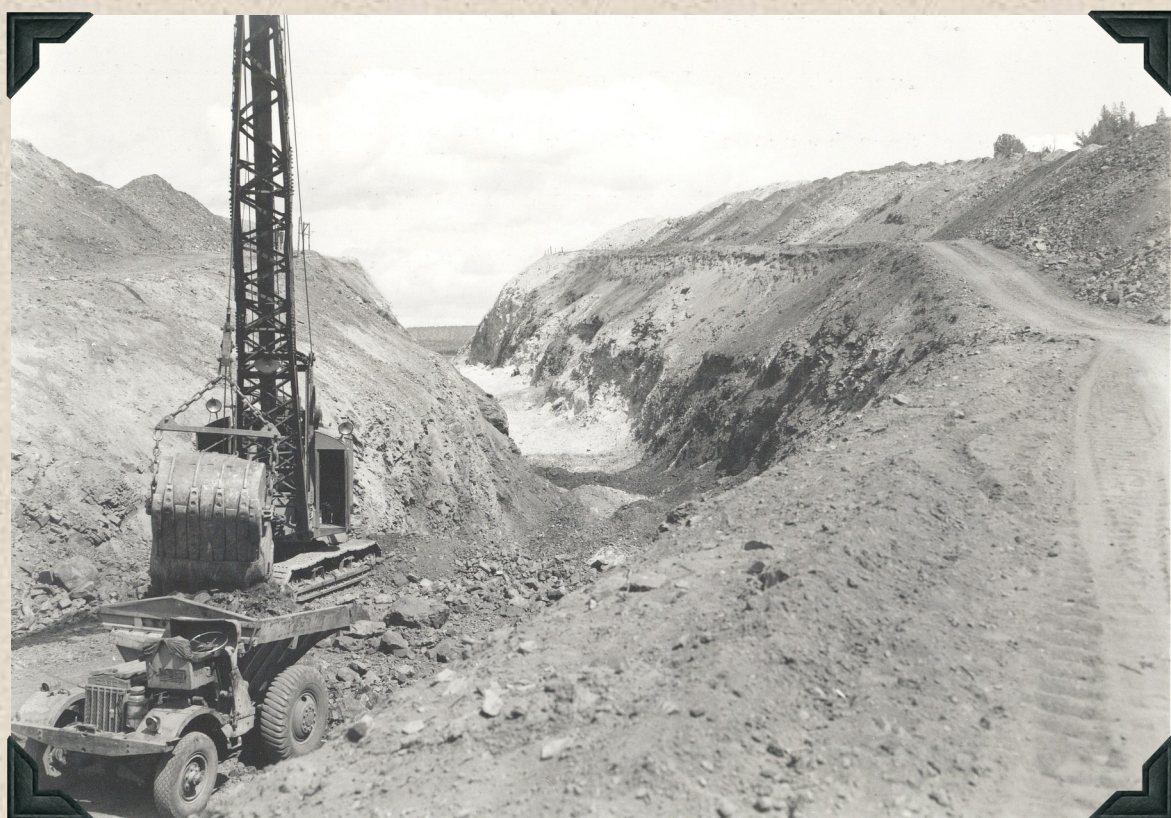
1942 - Looking downstream of North Unit Main Canal. "Big Cut" with approximately 20 feet of rock remaining.
