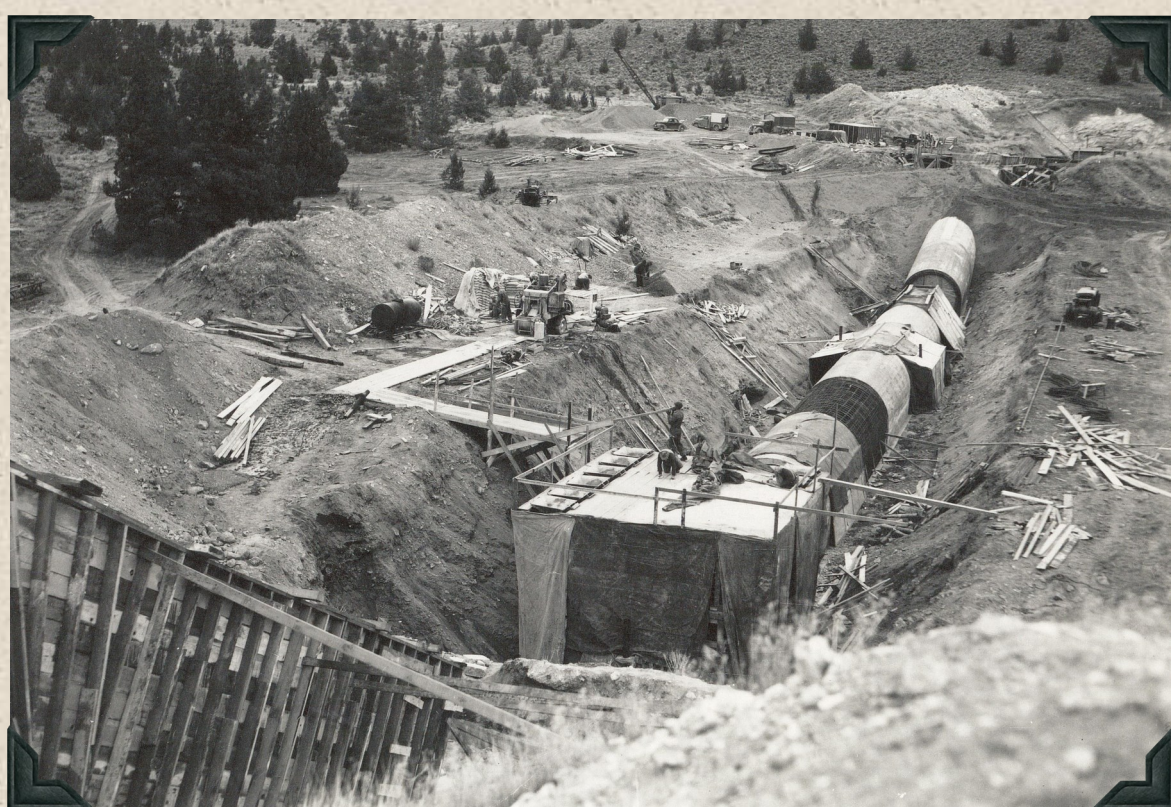
1945 - North Unit Main Canal. Sherwood Canyon Siphon, looking upstream. (McLaughlin Construction Co., Contractor)
