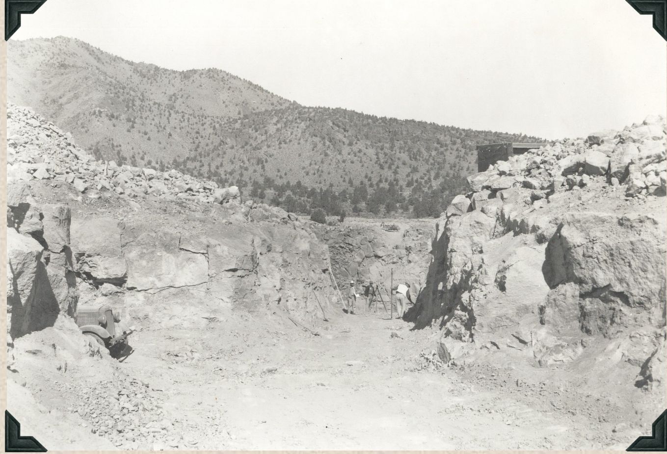
1944 - Rock excavation at inlet end of Crooked River Crossing, North Unit Main Canal.
