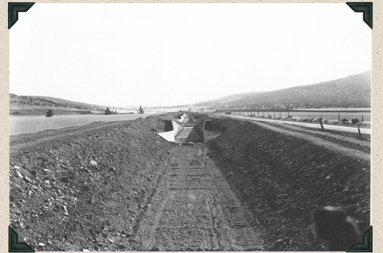
1945 - Lateral M-41, looking upstream from a bridge near Culver, OR. Six concrete drops, immediately after removing forms. North Unit Main Canal is visible at base of timbered slope on right and left. (Blickle & Cater, Contractor)
