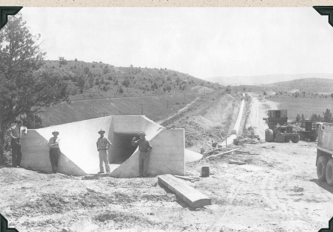
1948 - Lateral M-58. Inlet end of 54" concrete siphon, north of Madras, OR between Highway 26 and Highway 97.
