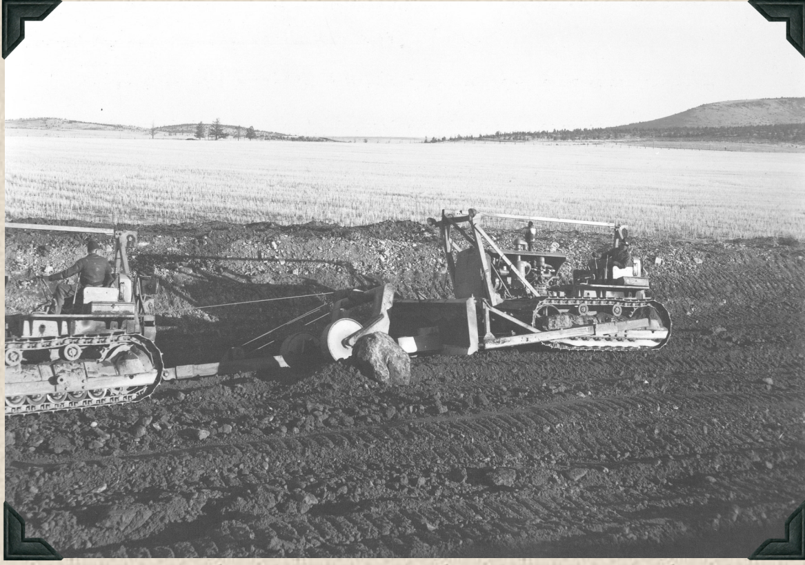
1942 - North Unit Main Canal. Side view of D-8 tractors pulling and pushing a single tooth ripper through hardpan material.
