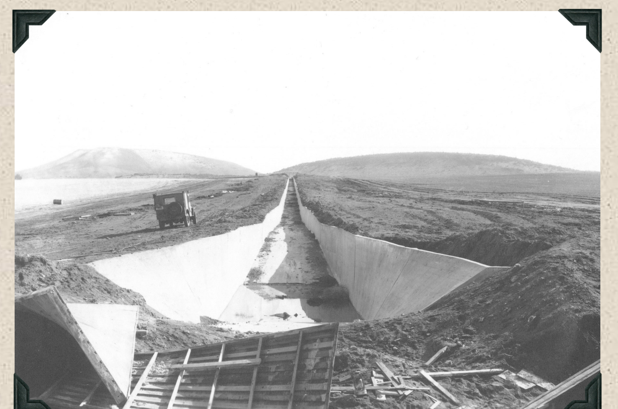
1946 - Looking upstream from foot plank on drop, Lateral M-43, showing concrete chute.
