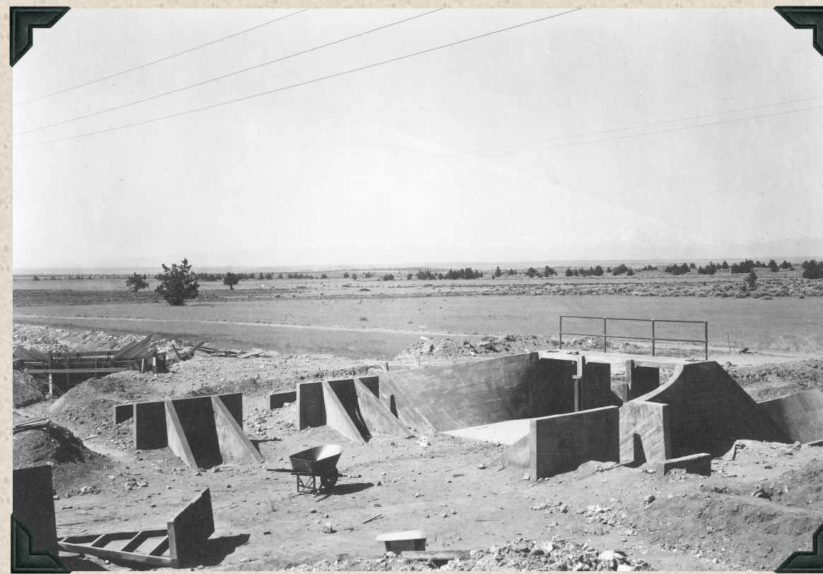
1945 - Lateral M-37 structures. From left to right, forms in place for weir drop on Lateral M-37-1, 24" turnout for Lateral M-37-1, 18" farm turnout to the left and weir visible just over transition wall, 18" farm turnout to the right, and check drop for Lateral M-37.
