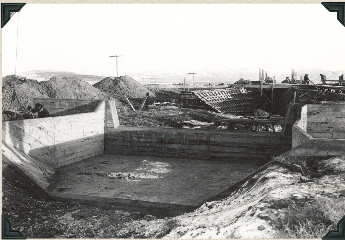
1945 - Lateral M-37 concrete structures. The "M" in M-37 represents mile. In this case the M-37 location is 37 miles downstream from the diversion in Bend.
